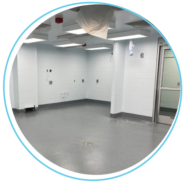
New dedicated ABSL-2 study space and stereotactic surgery suite are under construction at our Madison, Wisconsin site
